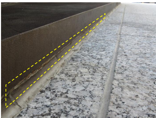
Figure 19. Corrosion product behind failed sealant.
