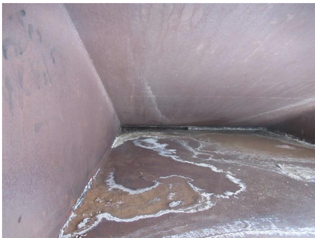
Figure 17. Salt deposits located in the back cavity.
